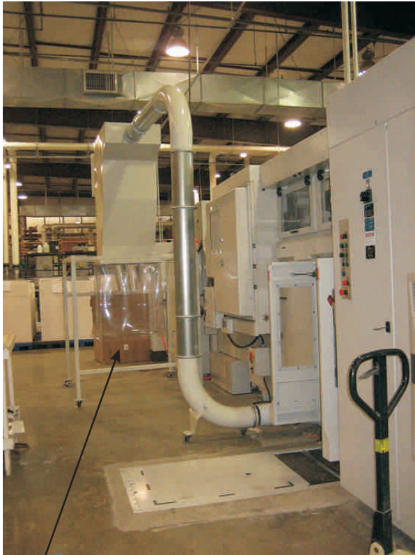
WASTE PAPER DISCHARGE AIR SEPARATOR SHOWN
